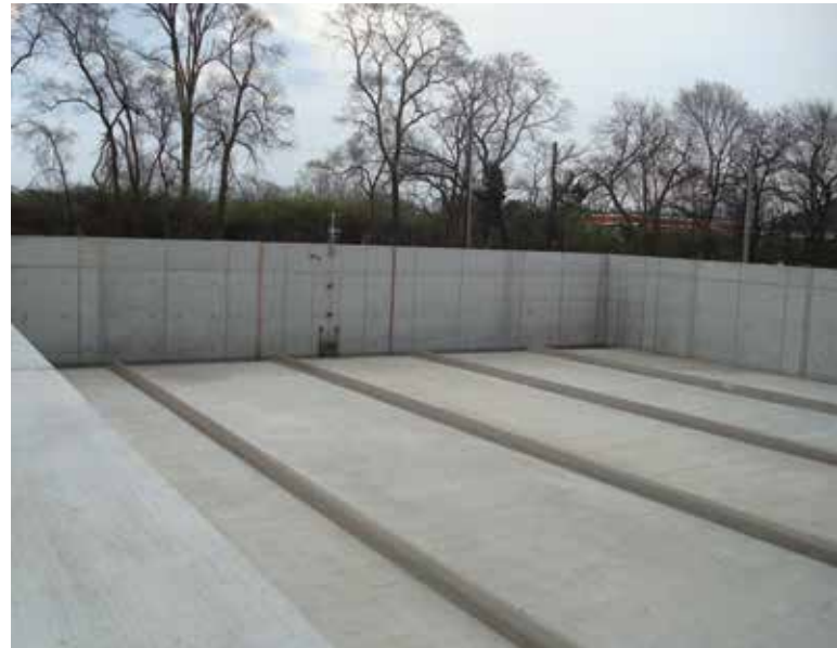
Wastewater Treatment Plant Flow Equalization Basin, Clyde, OH
