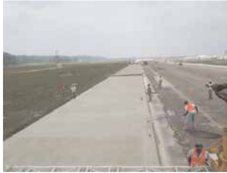
Airport paving at Spirit of St. Louis Airport in Chesterfield, MO, placed with blended cement (Type 1 (SM)) and Class C Fly Ash added separately.
