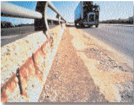
Figure 1: Penneable concrete is a principal reason for concrete deterioration due to reinforcing steel corrosion and other deterioration mechanisms.
